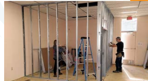
Contractors frame in a new private meeting space at the Forest Library location to support the integration of social services and provide a space for programming and community use.
