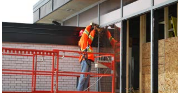
Workers remove the 60 year old window curtain wall as part of extensive renovations at Oil Museum of Canada in 2021.
