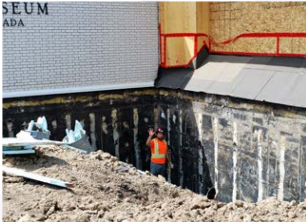
Workers apply a waterproofing membrane to the foundation wall of the Oil Museum of Canada as part of extensive renovations in 2021.
