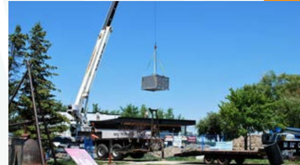
A new rooftop HVAC unit is lowered on to the roof of the Oil Museum of Canada as part of mechanical upgrades to the 60 year old building.
